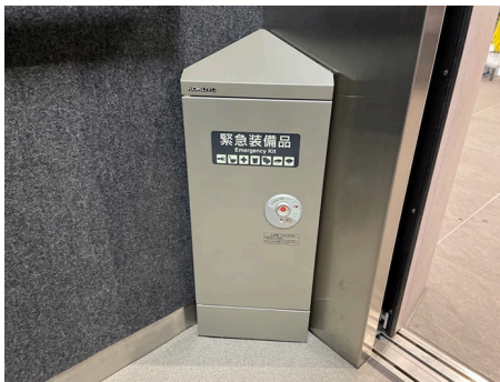
Installation of disaster prevention cabinet
