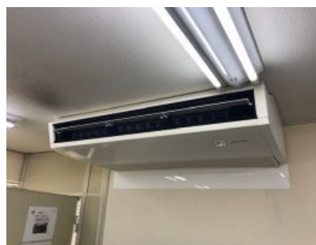
Update air-conditioning system
