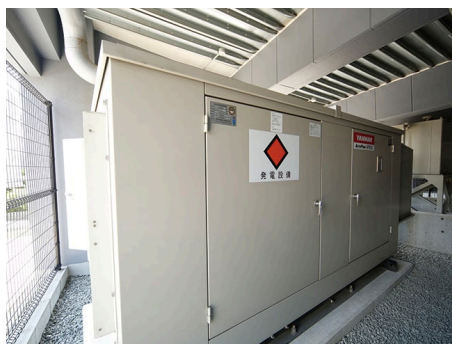
Installment of private power generators
