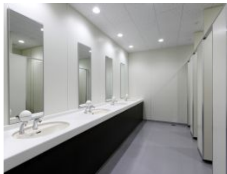
Installment of motion detected sensor
