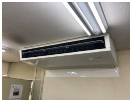
Update air-conditioning system
