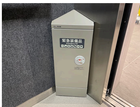
Installation of disaster prevention cabinet
